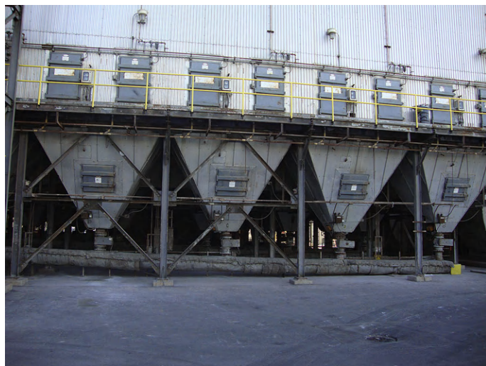
Figure 8.1 Typical fabric filter installation and fabric filter.
