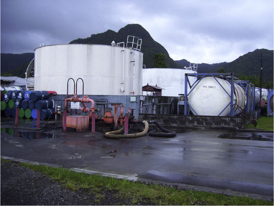
Figure 4.1 Waste oil holding tanks at ASPA power plant.
