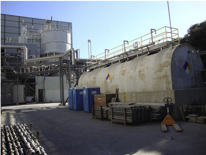
Figure 8.3 Installation illustrating use of ammonia tanks.
